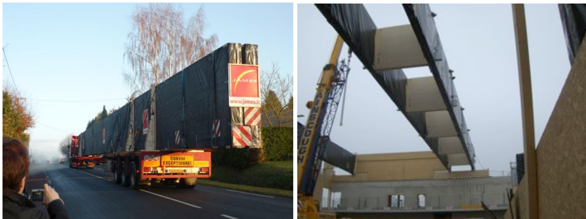
Figure 10: Eton Manor sports facility. Delivery and installation of main beams. Image copyright PJ Steer.
