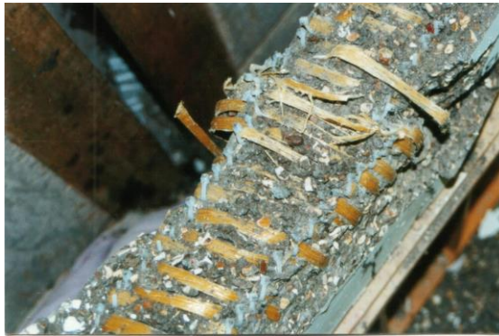
Figure 10. FRP helix ruptured at failure.
