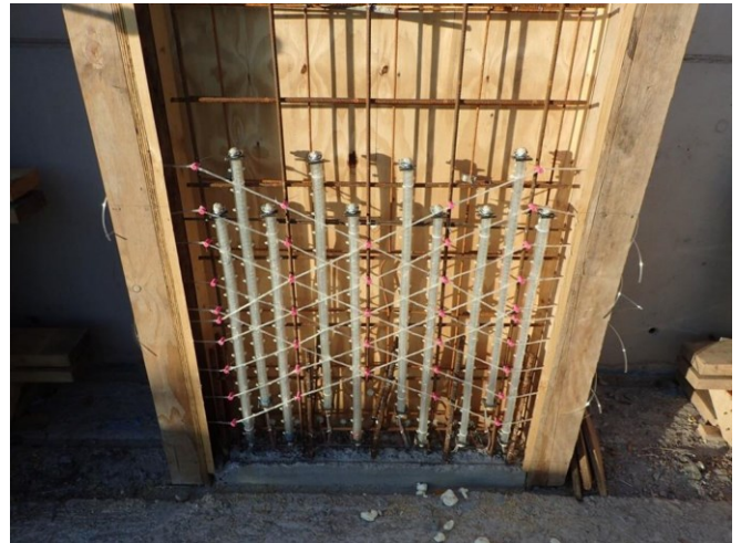
Figure 3: Shape memory polymers inserted at the base of a concrete wall (large vertical elements) and vascular network of tubes (diagonal elements) which will be removed after casting
