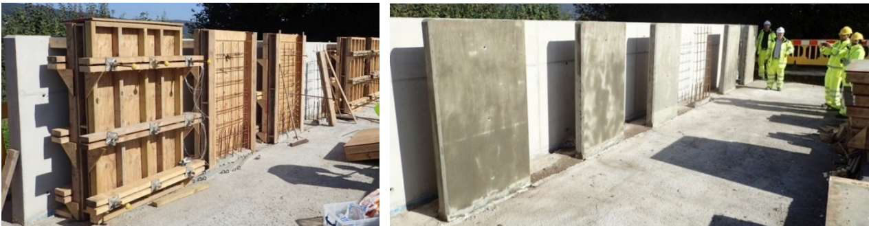
Fig. 6. The M4L field trials of self-healing concrete wall panels at the A465 site
