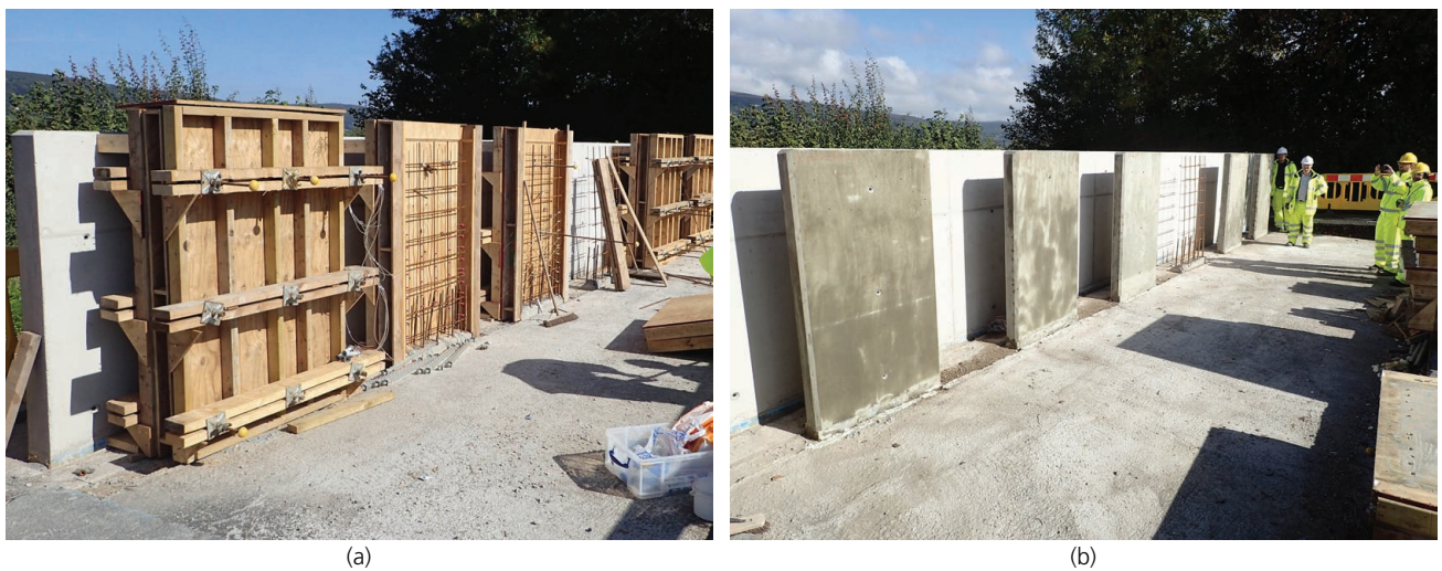
Figure 6. The M4L field trials of self-healing concrete wall panels at the A465 site (a) during construction and (b) after demoulding. Visible from left to right in both (a) and (b) are panels A, B, C, D and E. Details of self-healing systems are available in Table 1
