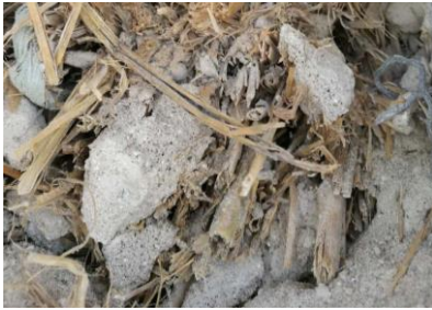
Figure 11. Mixture of straw and lime stucco outside the high position of laid flat bale wall
